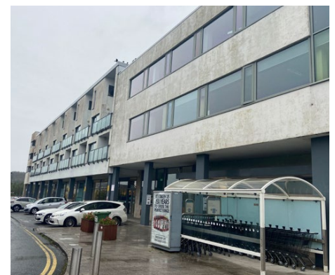
Development at Newtown Square is showing signs of wear, along with the block paved carriageway which is failing at key junctions due to stress by vehicles.
